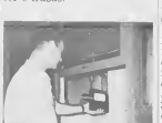
ERE'S INDUSTRIAL hygienist Richard S. Brief measures ventilation of laboratory hood with a device known as a Velometer.
